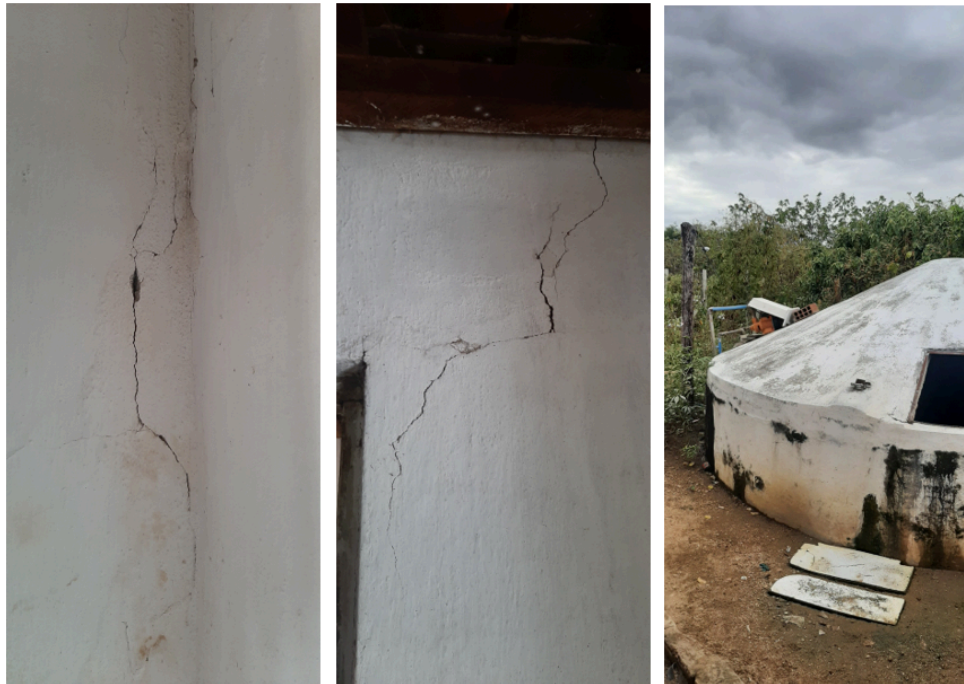
Figures 3, 4, and 5: Images of cracks recorded on the house walls and cistern of a resident of the Quilombola Pitombeira Community.
