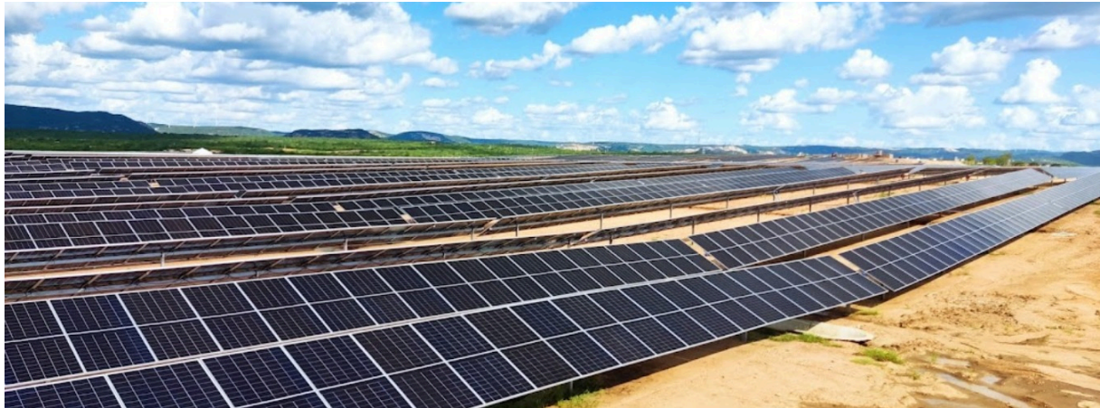
Figure 2: Partial panorama of the Luzia Solar Complex (Santa Luzia – Paraíba).
